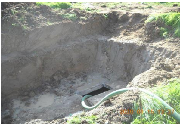
24.2-9.0 leak upstream of Rd. 22
