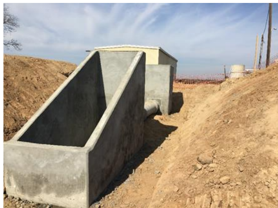
New turnout for Samran Farms on 6.2 Canal
