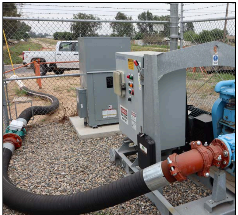
Ellis Basin Pump Station
